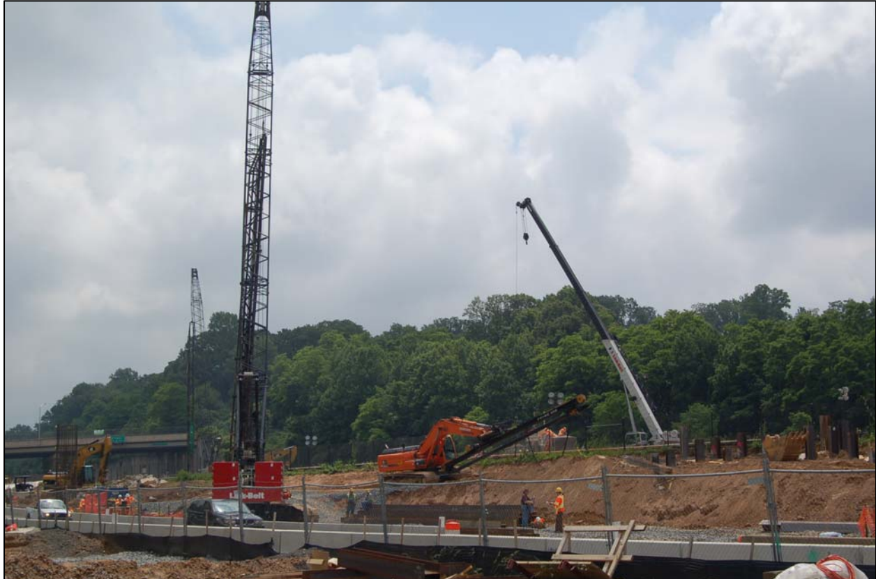
Dulles Metrorail Project construction taking place near the I-66/Dulles Connector Road interchange during the previous weekend.
